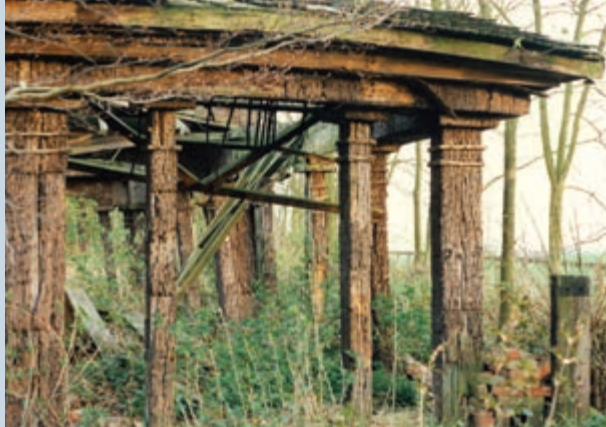
A side view of the surviving structure of the Bark Temple in April 1993. It finally collapsed during the winter of 1997/98 (SS)
