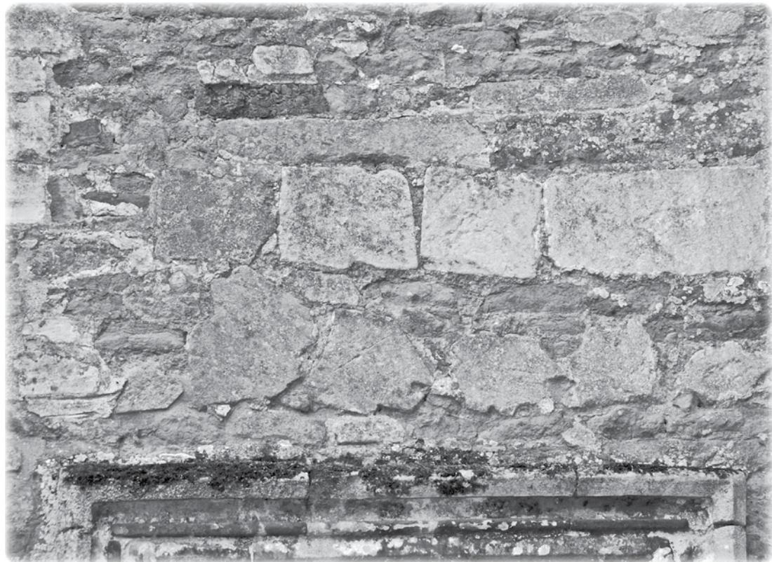
Example of repair work using recycled stone window mullions - Langham Church north chancel exterior wall - Photo Mike Frisby
