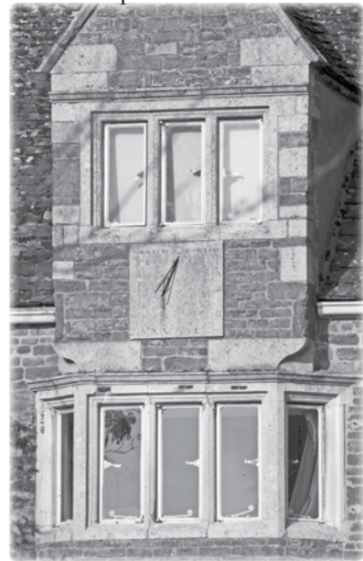
Langham - The Manor Detail of the stonework between the 1st floor bay and 2nd floor dormer windows
