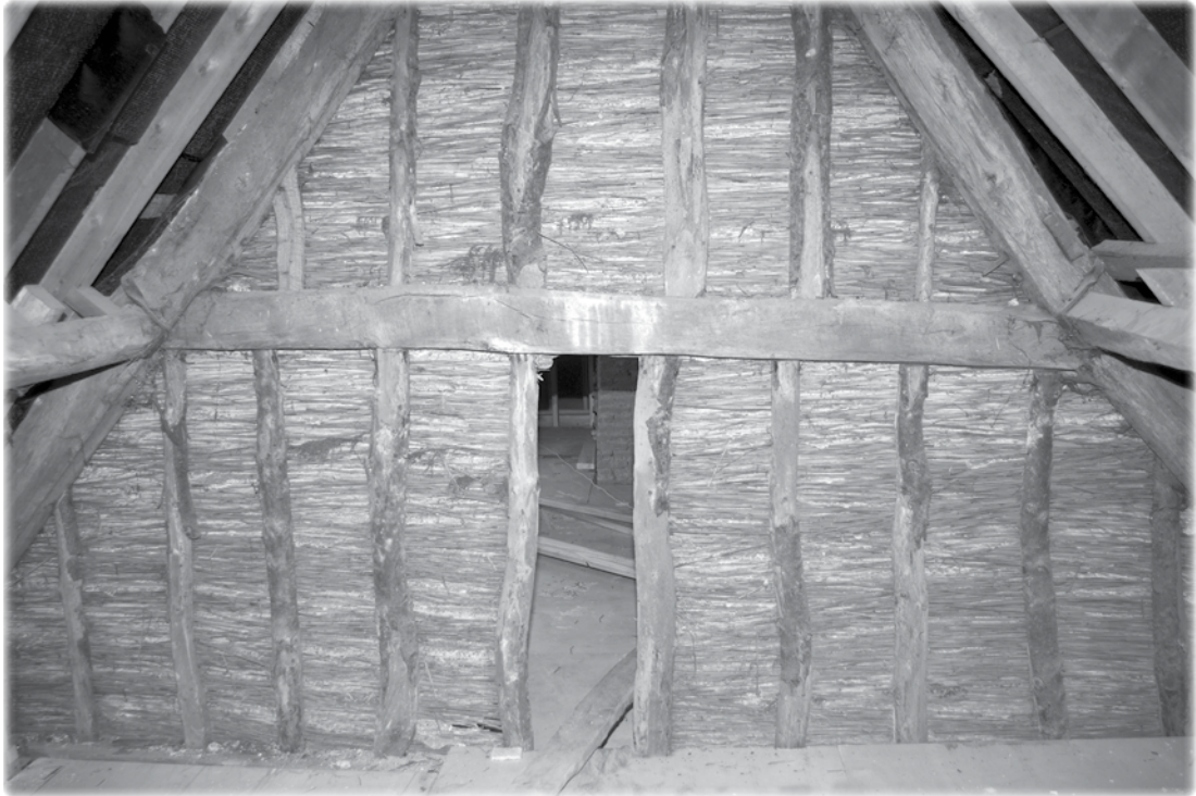
Well Street 15th century house - A main roof truss with timber and reed partitioning - Photo Mike Frisby
